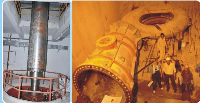
Godavari Lift Irrigation Scheme, Phase II, Andhra Pradesh Metallic Volute Pump - 25200 cum/hr x 131 m x 12.8 MW
